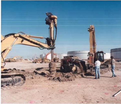
Liquid Storage Tanks, Houston, TX
