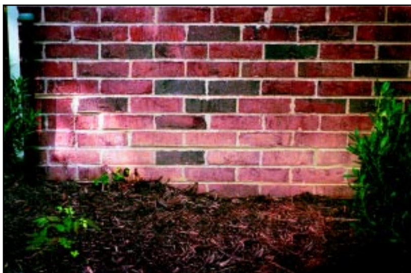
After HELICAL PIER® Foundation Systems stopped the foundation from sinking. Mortar repairs now will have a chance to last, too.
