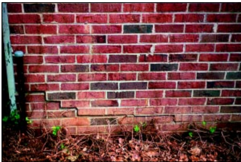
Before Typical "stairstep" cracks in mortar indicate the deeper cause . . . foundation settling problems.
